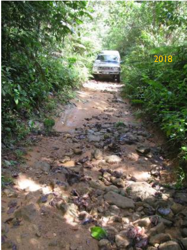
Photo 4: Badly eroded sections of the road in 2018 prior to renovation (Photo: Prof IAUN Gunatilleke)
